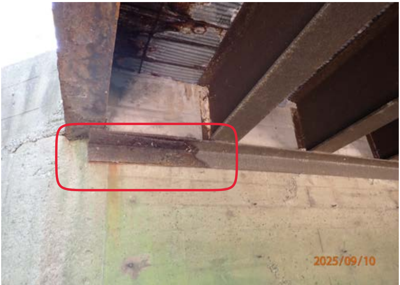
Metal support braces at exterior beams heavy corrosion
