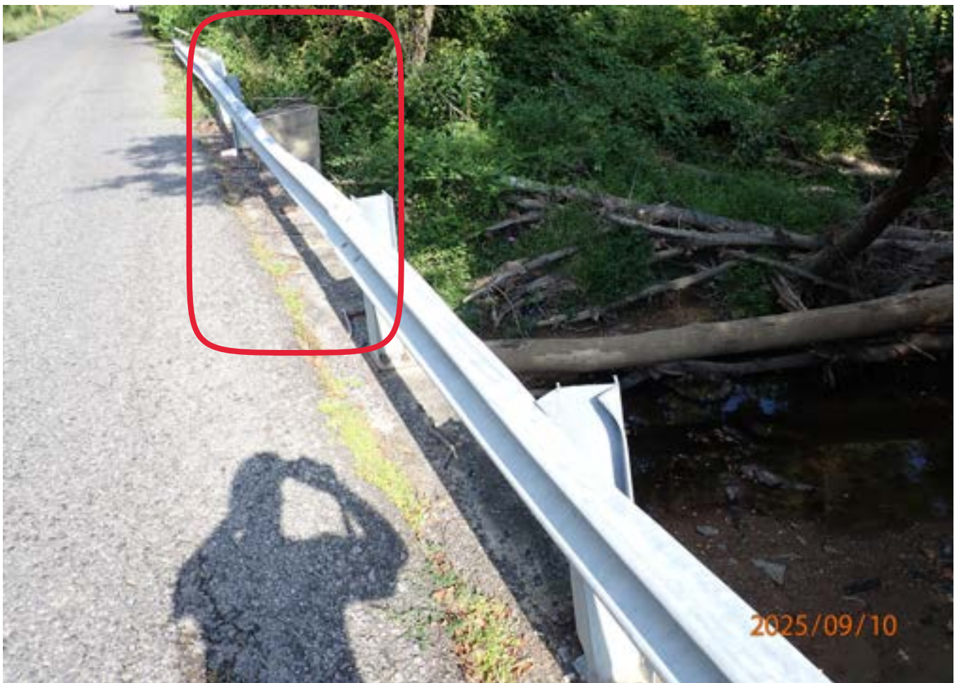
Downstream rail - damage near midspan towards ab 1
