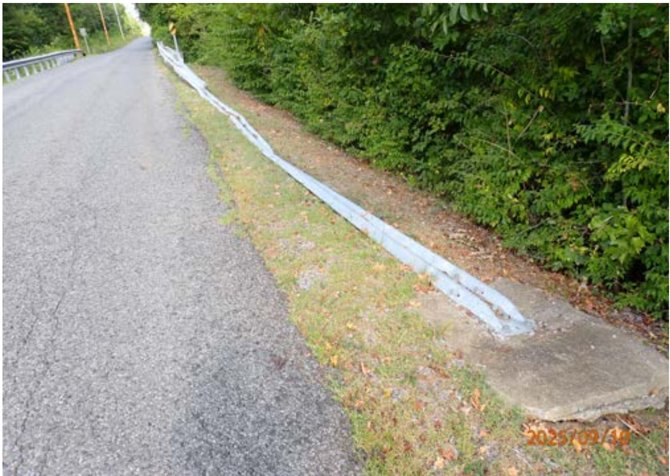
East transition rail laying on the ground (Damage)
