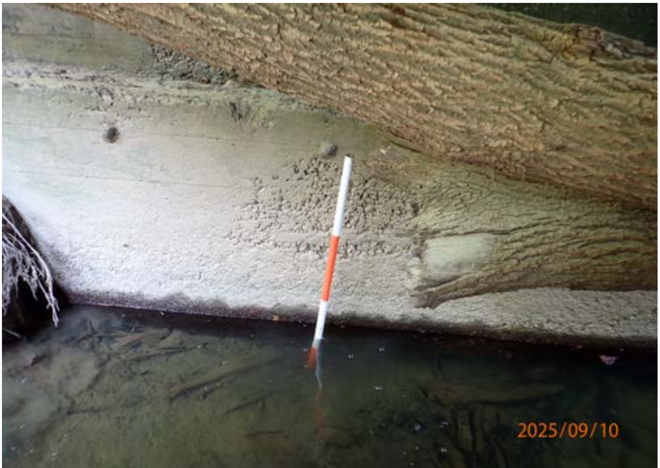
Abutment 1 - vertical scour up to 1' below footer
