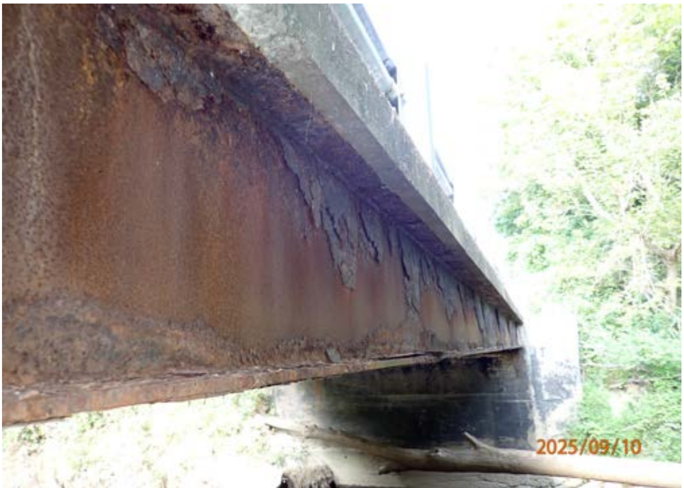
Beam 1 flaking rust is present with measurable section loss
