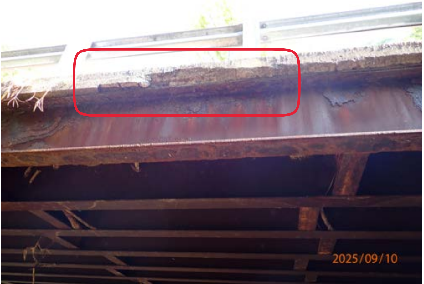
Upstream concrete over hang spall with exposed steel CS 3
