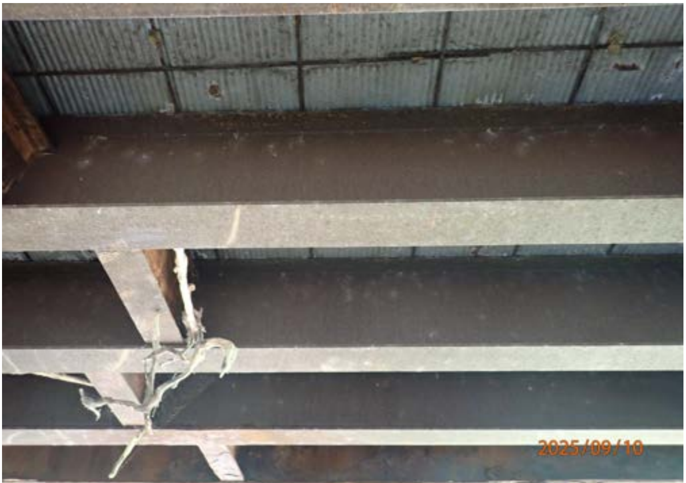
Typical of CS 3 corrosion on all beams
