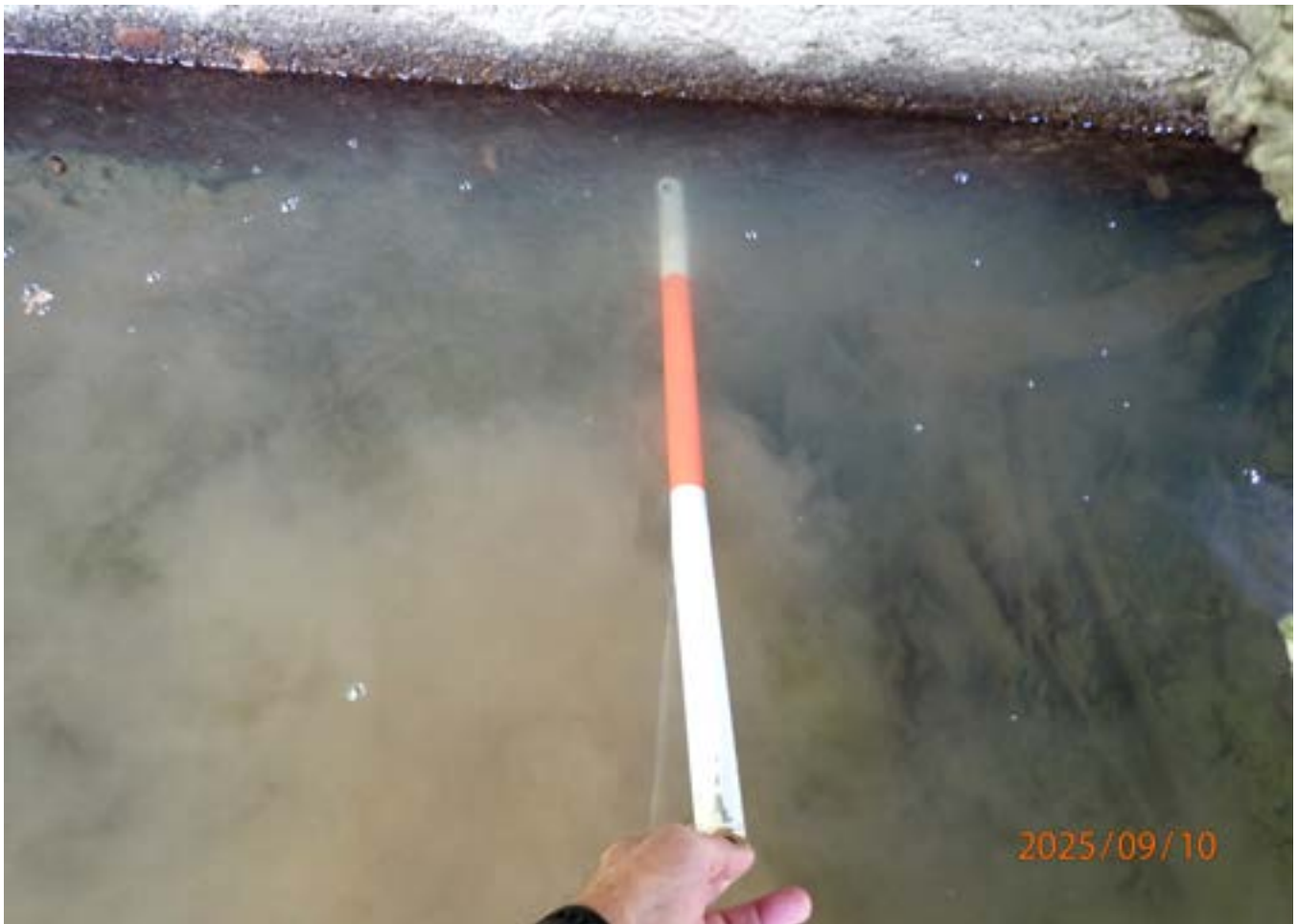
Abutment 1 - horizontal undermining up to 1'
