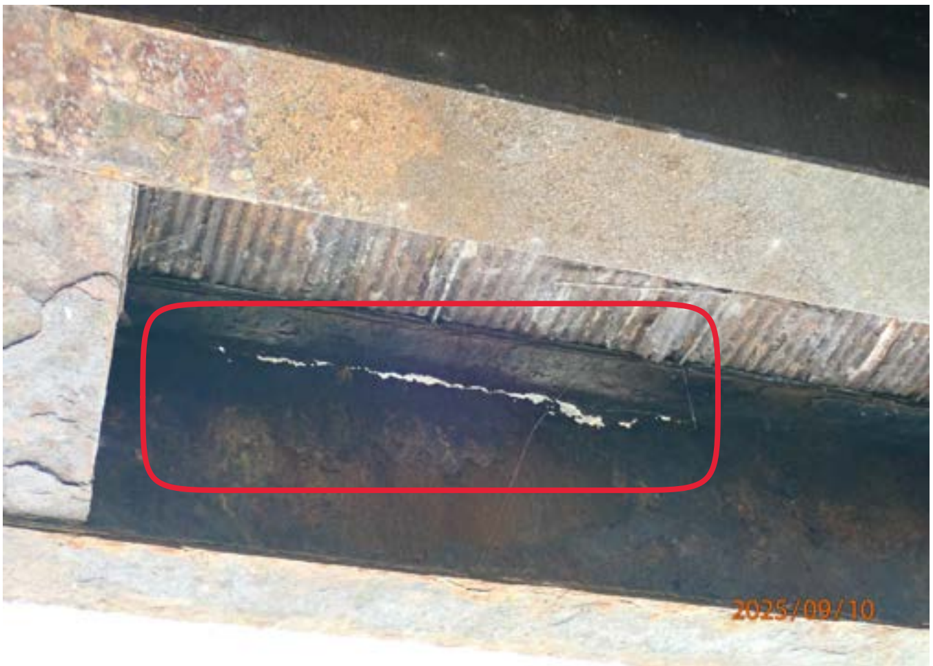
Beam 8 has a corrosion hole 3' long and 1.5 " tall CS 4 = 3'
