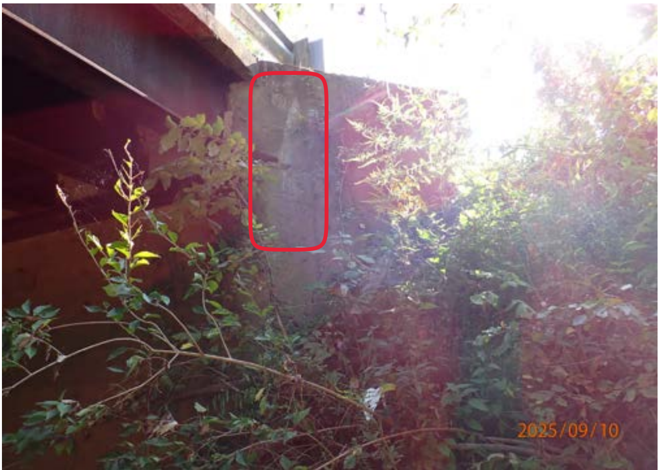
Cracking with leaching on abutment 2 wing wall
